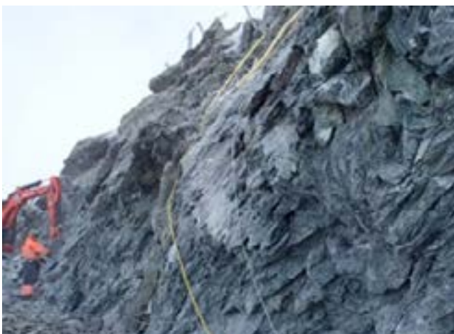
Strongly foliated serpentinite at the excavation front. (b) Typical superficial undulated rock flakes
