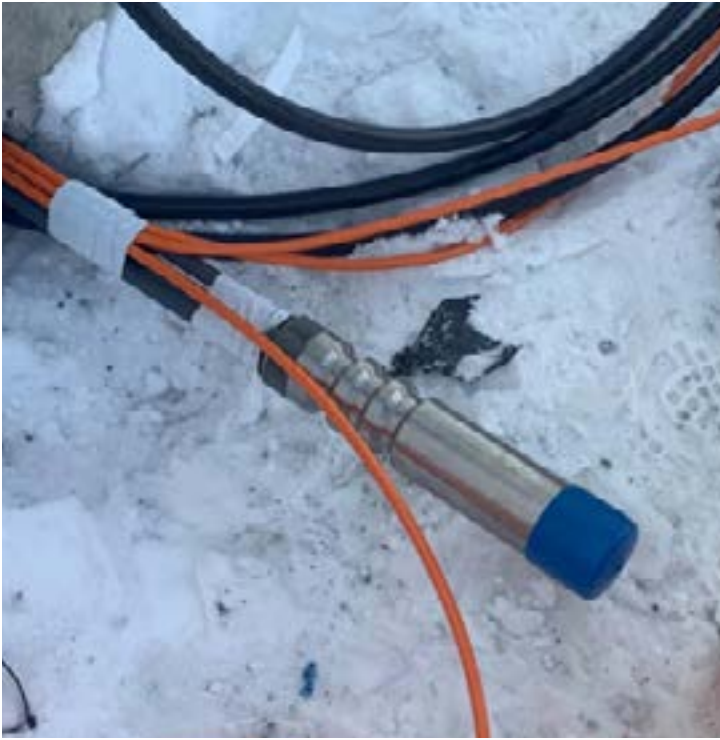
Borehole extensometer head (type Huggenberger) with cables of temperature string
